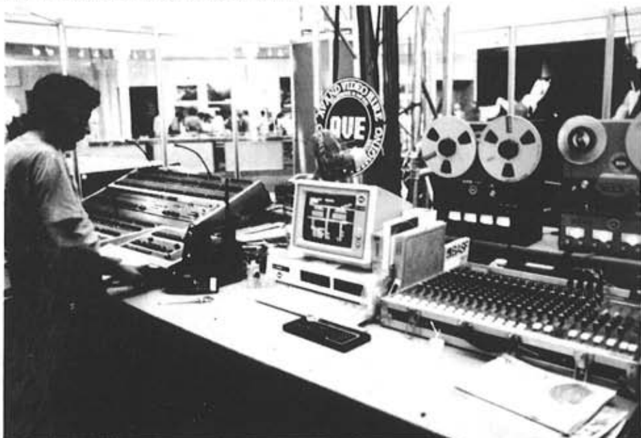
Inside the central control room, where the audio, projection system and lighting controls are located. Several audio visual shows were running around the perimeter of the dome.
